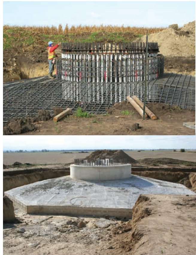
Figure 2. The construction of a utility-scale wind turbine foundation in Benton County, Indiana.
